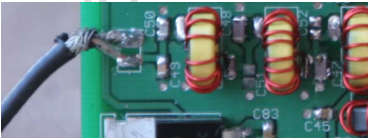
Figure 63. Antenna coax connection to transceiver. Upper connection is ground, lower is antenna.
